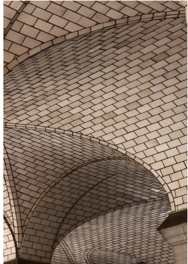
Vaulted ceiling with Guastavino tiles, Manhattan Municipal Building, New York City, completed in 1914.
