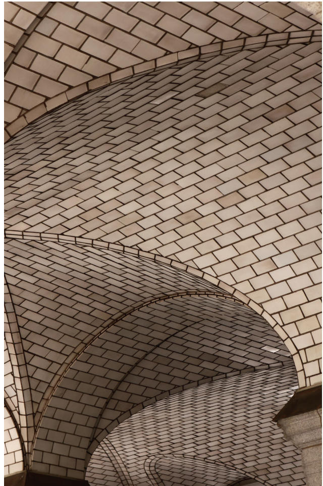
Vaulted ceiling with Guastavino tiles, Manhattan Municipal Building, New York City, completed in 1914.
